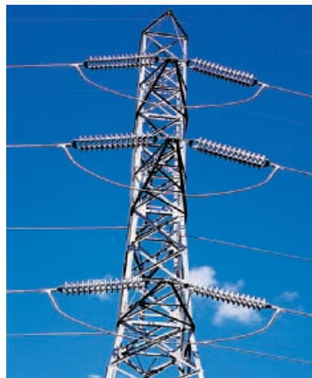
These high-voltage transmission lines are made of aluminum supported with steel cables.
